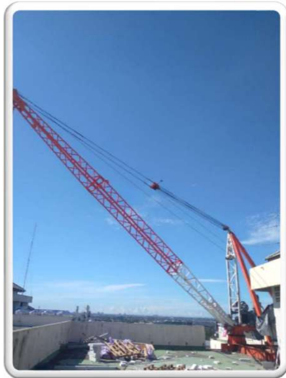
Derrick Crane No.11
