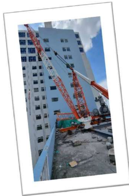
Derrick Crane No.12
