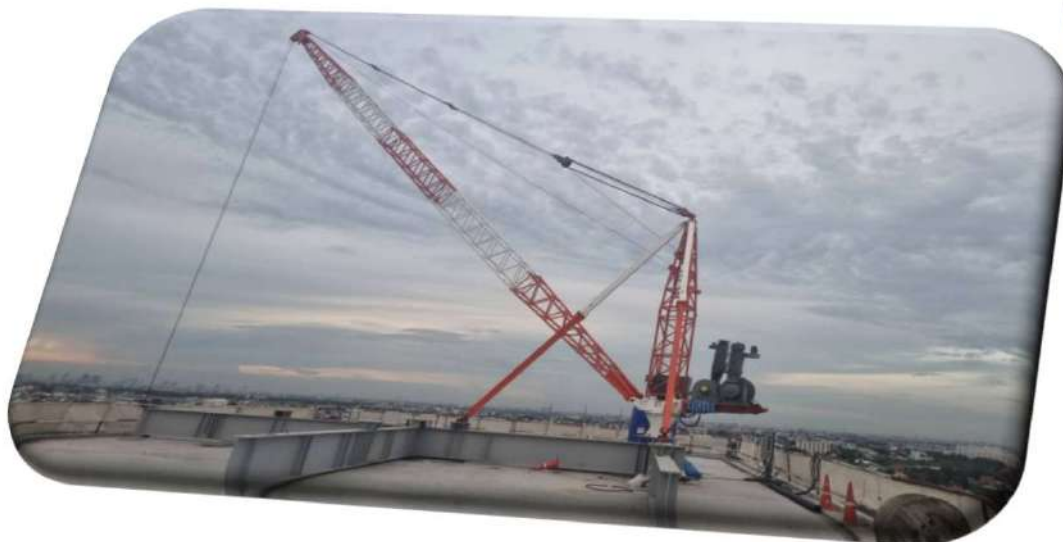
Derrick Crane No.7
