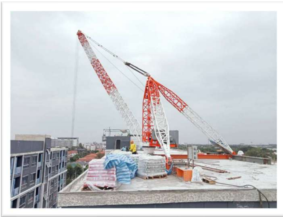
Derrick Crane No.5
